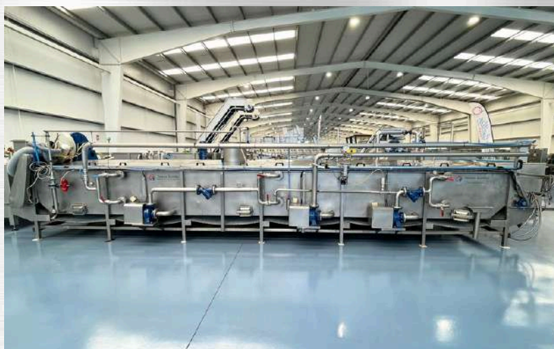
IN-LINE COOLING TUNNEL
